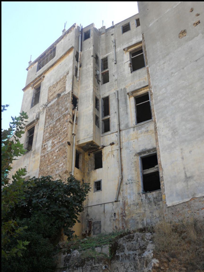
158 damage from civil war
